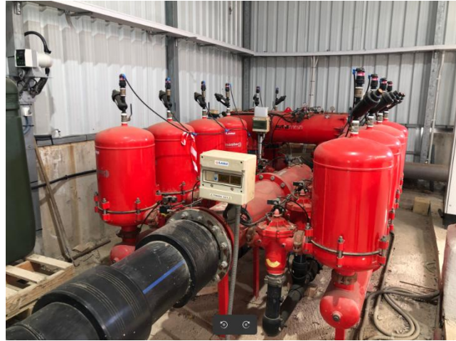
Figure 3-61: Mesh filters for tertiary treatment at Algarrobo irrigation association
